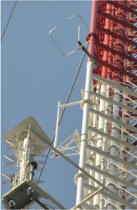
Looking from the transmitter building with the top of the Ch. 9 standby antenna at the bottom.
